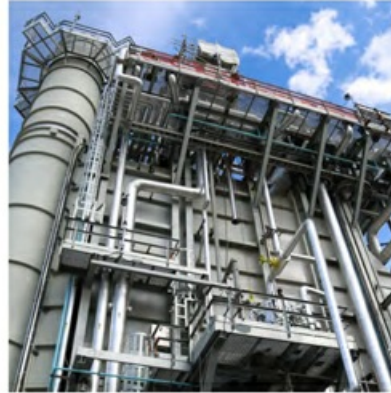
ExxonMobil has interests in more than 100 cogeneration facilities around the world, with the latest unit recently completed at Imperial's Strathcona refinery in Alberta, Canada.
