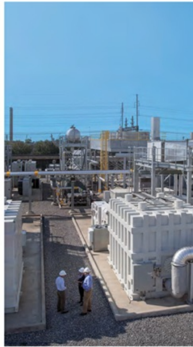
FuelCell Energy reports its 14.9MW fuel cell platform in Bridgeport, Connecticut, has provided clean and reliable power since 2013.
