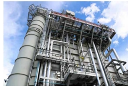
→ ExxonMobil has interests in more than 100 cogeneration facilities around the world, with the latest unit recently completed at Imperial's Strathcona refinery in Alberta, Canada.
