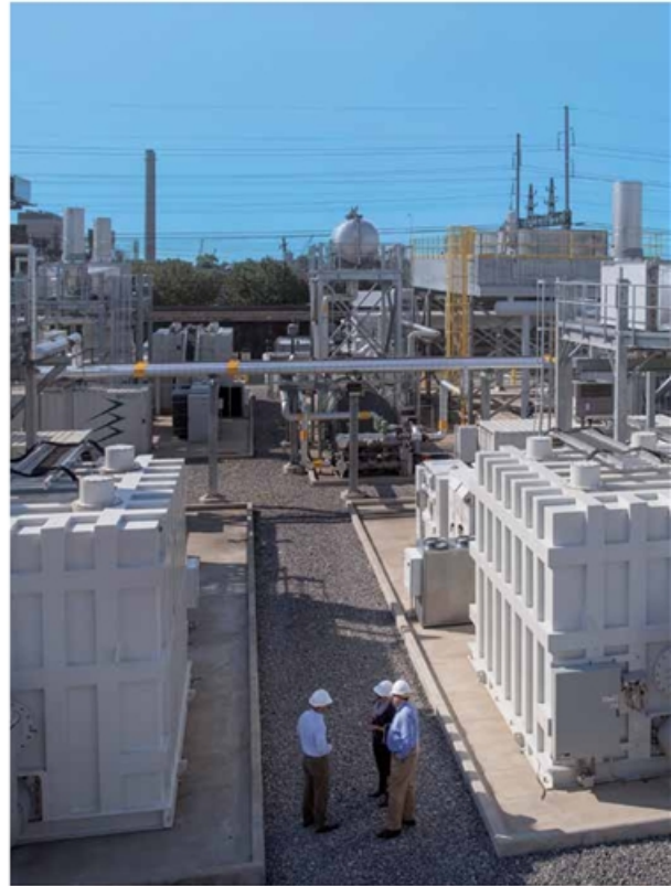
→ FuelCell Energy reports its 14.9MW fuel cell platform in Bridgeport, Connecticut, has provided clean and reliable power since 2013.
