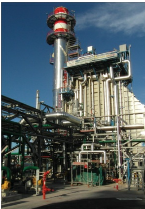
Our newest cogeneration facility at our Augusta Refinery in Italy was commissioned in 2013. These highly efficient facilities provide a significant portion of the energy to our refineries.
