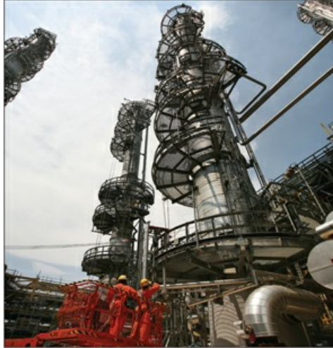
Our Singapore Expansion project installed extensive heat integration to improve energy efficiency and lower cost.
