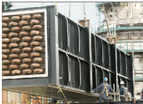
A new furnace is installed in the vacuum distillation unit of the Dartmouth refinery in Nova Scotia, Canada. This project will increase capacity and reduce energy usage.
