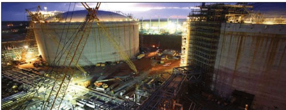
Construction progresses on the South Hook LNG regasification terminal in Milford Haven, Wales.
