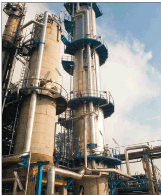
Upgraded facilities at our Treccate, Italy, refinery are one of several ExxonMobil projects that increase conversion and high-value product production.
