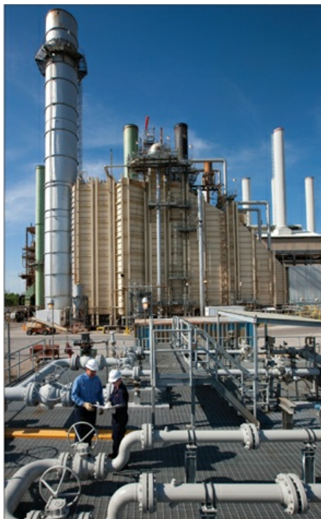
The Baton Rouge Refinery's cogeneration unit generates enough electricity to fully power the complex plus 30,000 homes on the regional power grid.
