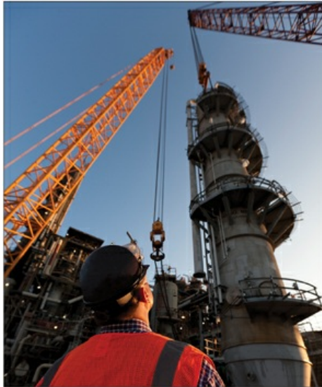
In 2011, our Baton Rouge chemical plant installed new facilities to further expand feed flexibility.
