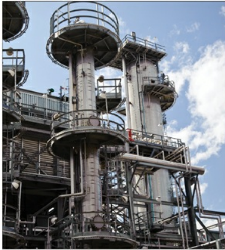
Comprehensive global management systems are applied in projects and operations around the world, including at our Strathcona Refinery in Alberta, Canada.
