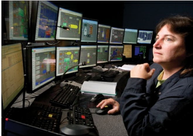
Specialized training and well-equipped control rooms are essential components of operational excellence.
