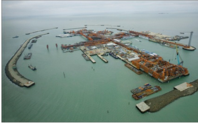
The Kashagan project facilities are 95 percent complete, and drilling is progressing according to plan.
