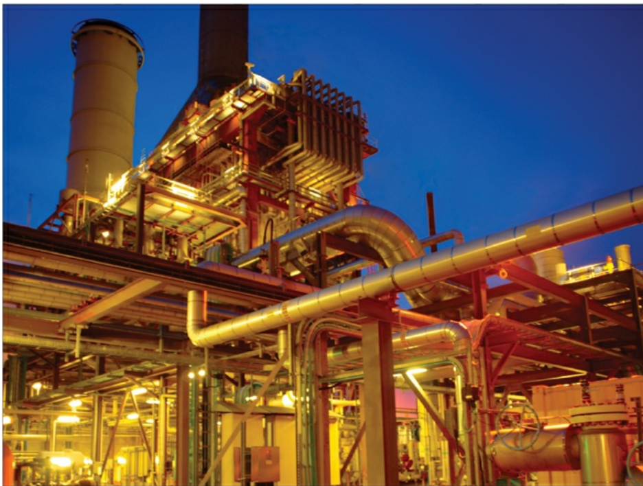
Cogeneration provides a significant source of efficient energy for our refining and chemical sites. In 2010, we purchased a 125-megawatt cogeneration facility to more efficiently supply steam and electricity for our integrated facility in Fawley, United Kingdom.
