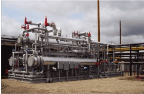
This testing equipment was installed at the West Pembina field in Canada to conduct a field trial of ExxonMobil's proprietary ColdFlow technology, which combats the formation of hydrates.
