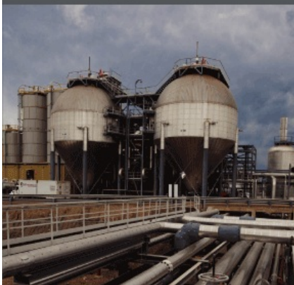
Water recycling units installed at the Cold Lake project in Canada allow 95 percent of the project's water to be reused.
